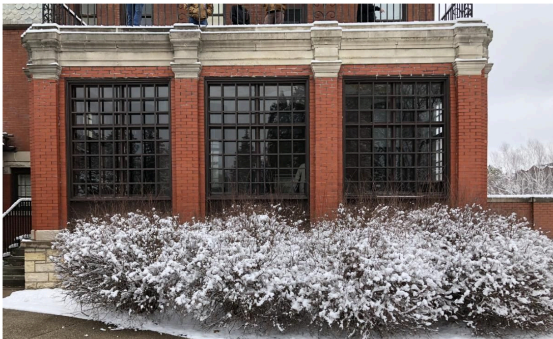
This wooden trellis system, also fabricated from Accoya, was a giant part of the renovations. The pieces ranged in size from 104" x 93" to 80" x 93". The joints were ship-lapped and placed in front of windows to match the previous trellis faithfully.
