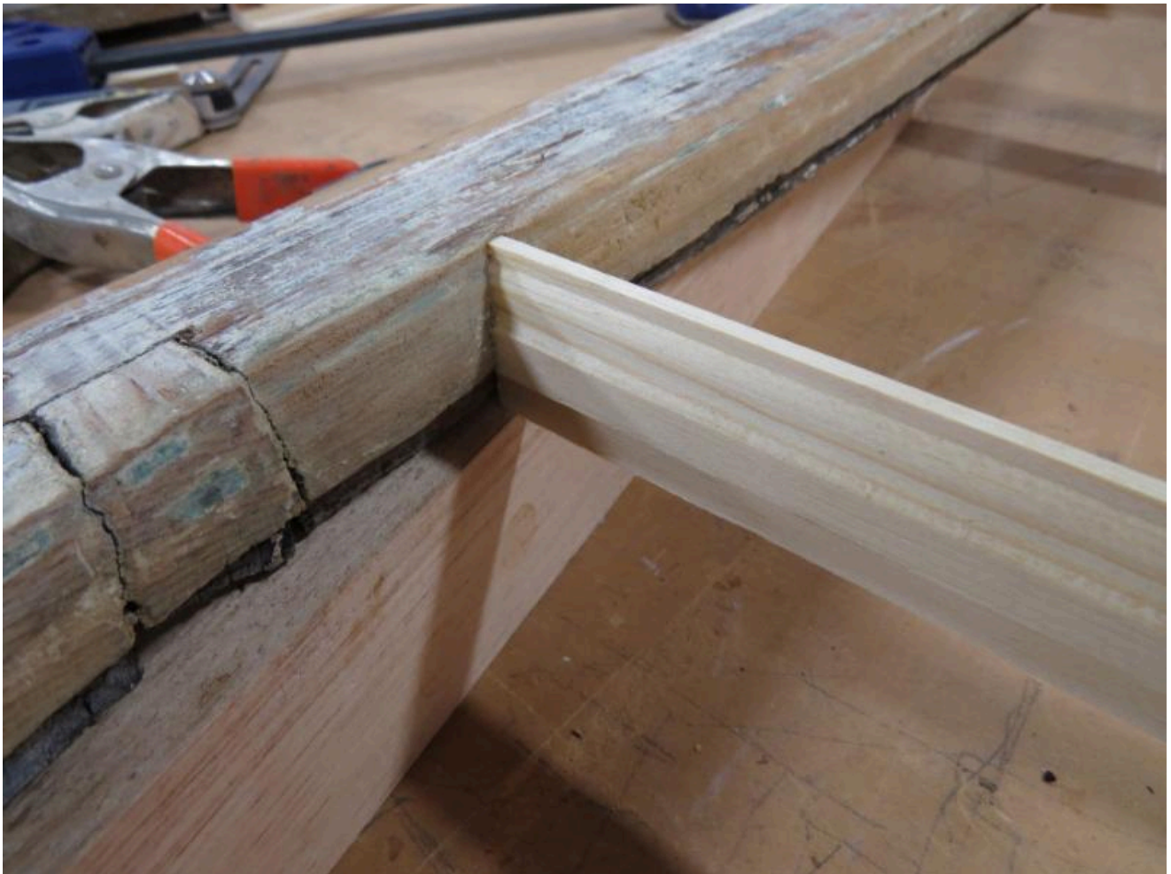
In this close-up, the new muntin bar was joined to the stile of the window sash. Our shop takes pride in making the joints fit tight even though the profile is almost gone on the original window.
