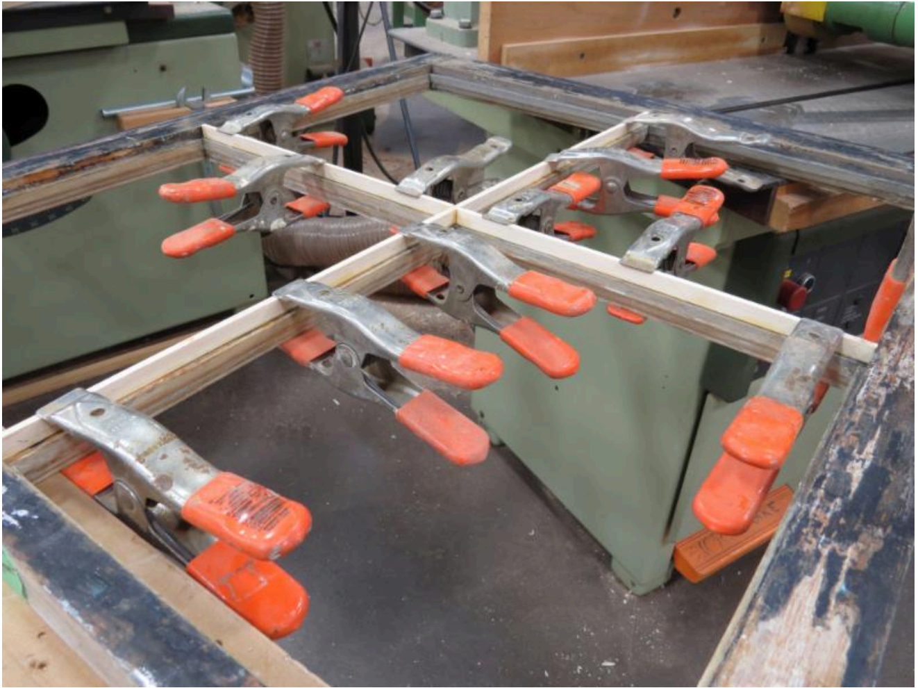
Replacing the web on the muntin bar in depicted here. The web is the part of the muntin bar that holds the putty and the glass in the window sash.
