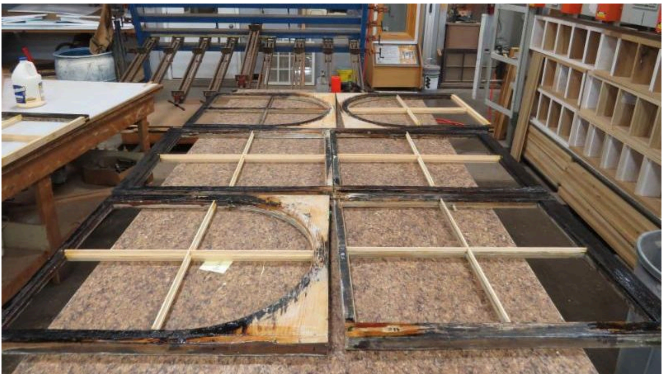
Three complete window sash sets in the early stages of repair. You can see that the muntin bars
