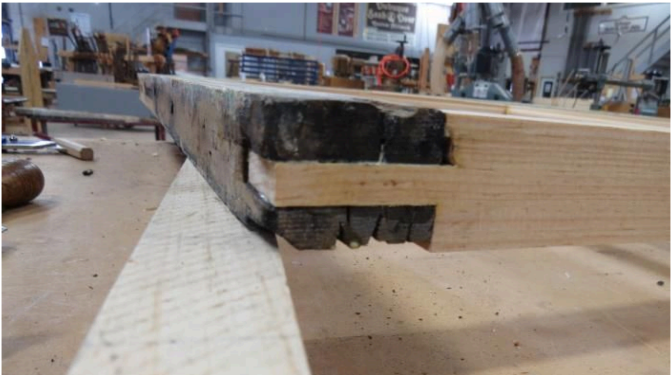
A close-up picture showing the mortise and tenon joint between the new bottom rail and the original stile of the window sash. The pieces will be fastened together and epoxied to create a tough joint.
